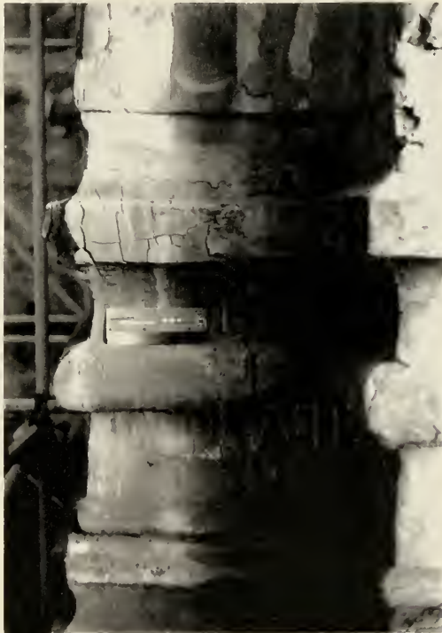
Fig. 28. Open and defective joints at base of pilaster at the intersection of the east transept and east wall of nave (Photo: Anne Brackin).
